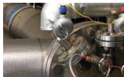
Used at a commercial Sustainable cooling for a warming planet heating loop in Juneau, Alaska, to generate hot water, reaching temperatures of over 100c and reducing the use of 7,775 gallons of diesel per month.
