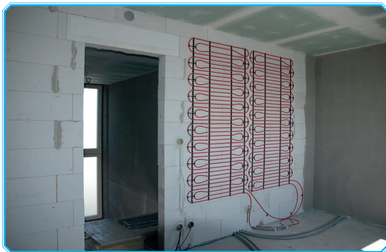
Picture 26: Low temperature heating and cooling in a passive house (Hviezdoslavov) before plastering (Slovakia)
